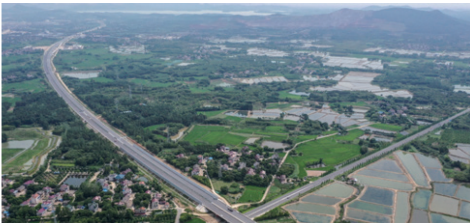
A section of the Liyang-Ningde Expressway, connecting Liyang of Jiangsu Province and Ningde of Fujian Province, under construction on July 26, 2022 (XINHUA)
