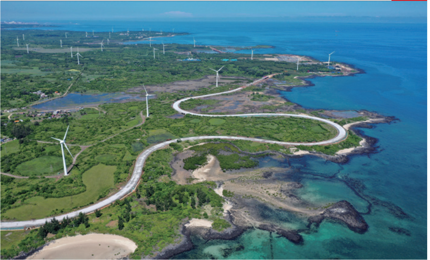
Construction site (drone photo) of the Danzhou section of Hainan's round-the-island tourist highway on July 23, 2022 (XINHUA)
